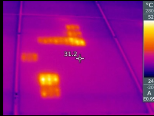
Hot spots resulting from micro cracks damaging the cell structure
